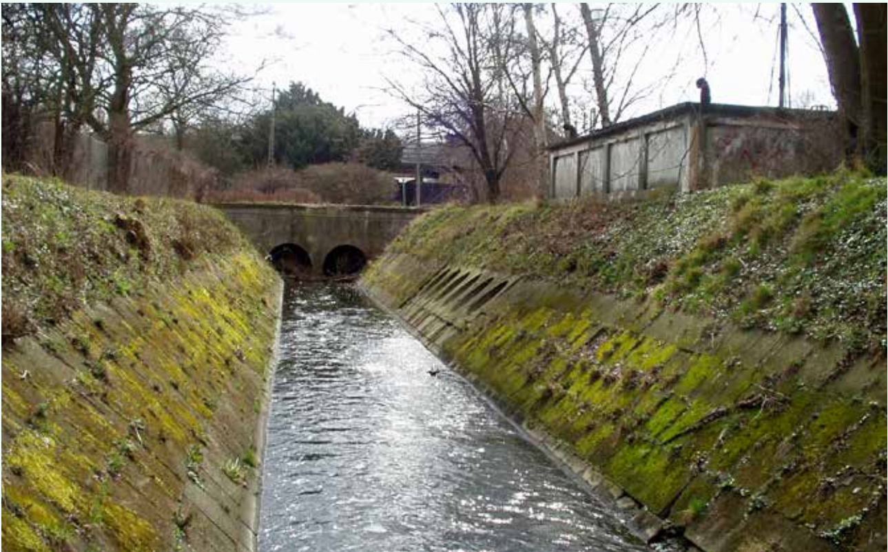
In the future, citizens will benefit from the streams expansion making room for more water during heavy rain. Photo by Jan Burgdorf.
