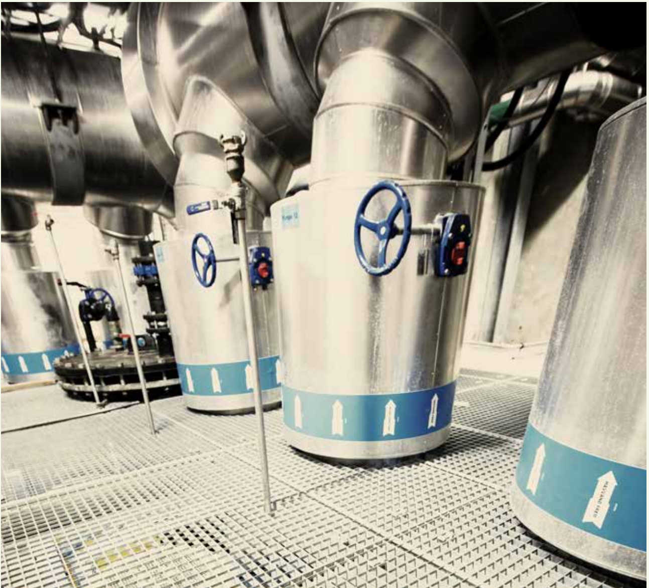
Pumps in the cooling plant in Adelgade in the inner city of Copenhagen. Photo by HOFOR.
